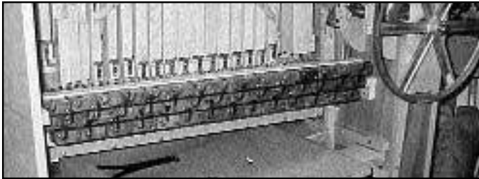
Figure 40. A view of the three rows of valves mounted on the pneumatic chest.
